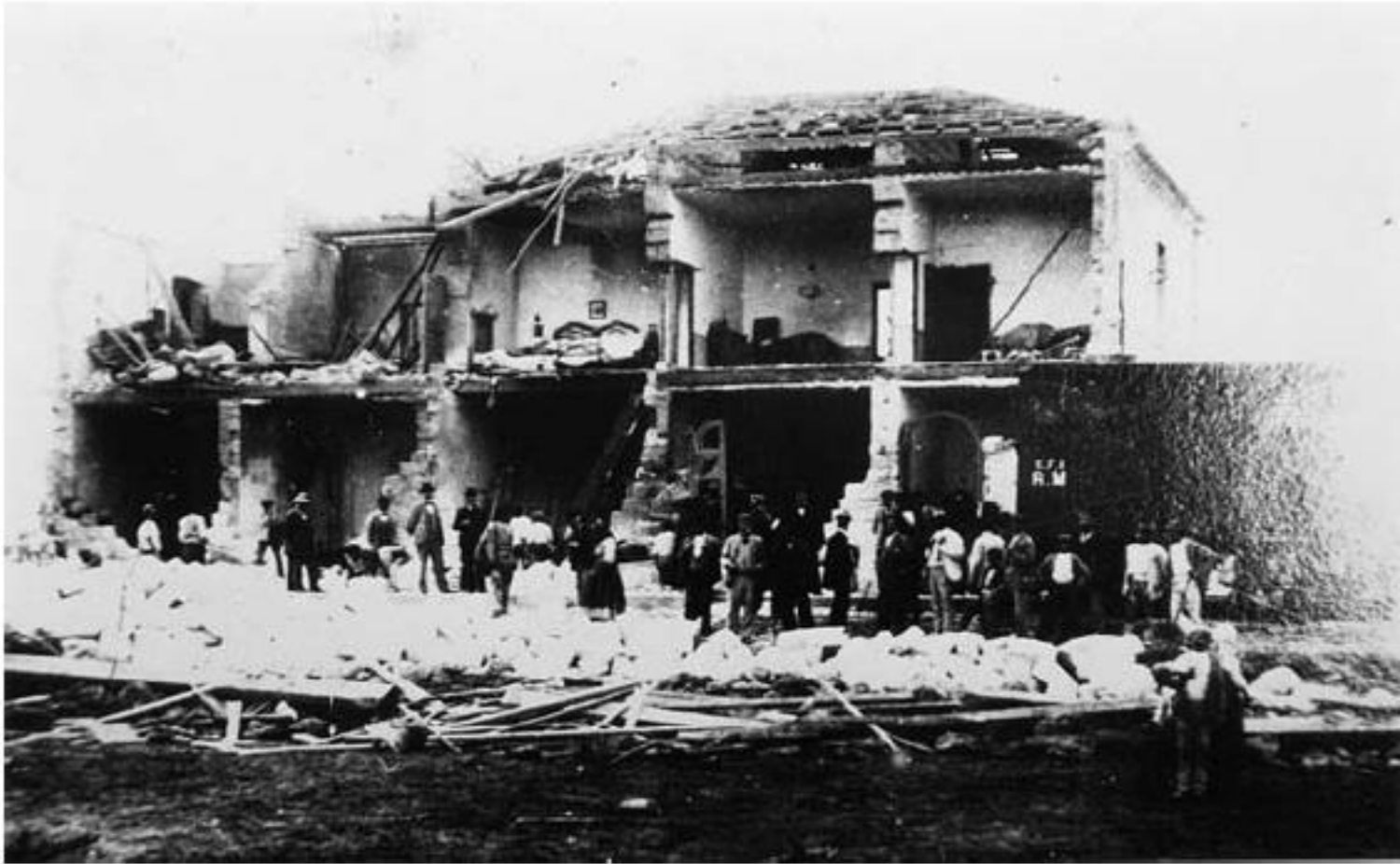
Photo 2. Oria. A view of damage produced by the 21 September 1897 tornado on houses placed near the railway station.
